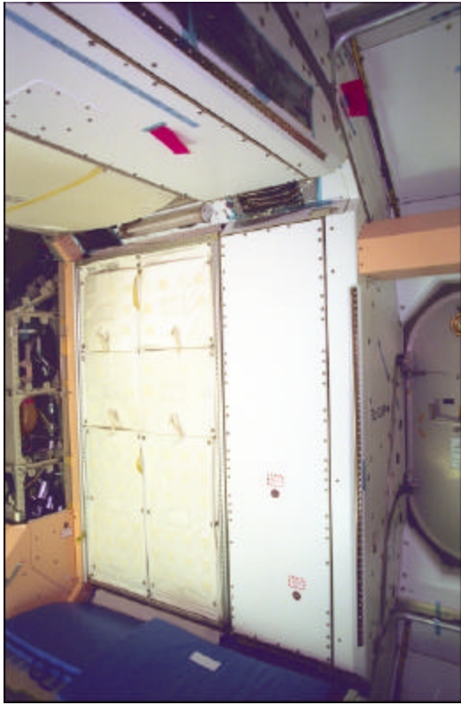
ZSR installed in the Unity Node
