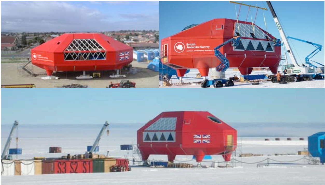
Figure 9. Central module showing test erection in Cape Town (top left), under construction on site with pre-glazed panel being lifted into place (top right) and nearing completion (bottom)
