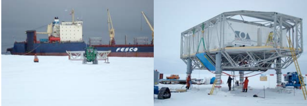
Figure 6. Space frames were unloaded from the ice strengthened Russian vessel, Anderma , and dragged across the sea ice using lightweight transit skis. Once at site (right side) the hydraulic legs and permanent skis were installed, followed by prefabricated services, floor cassettes, prefabricated room pods and the superstructure
